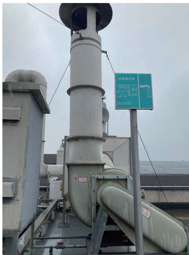
The exhaust gas treatment facilities of NJCTT
